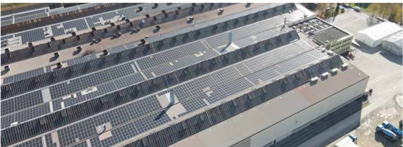
Fig.: PV system on roof of seamless tube rolling mill
