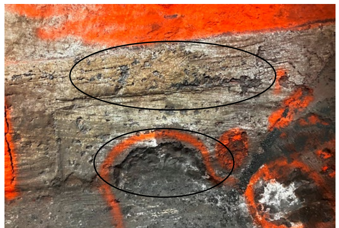
Figure 7: Close-up of a nickel chute. Note the surface defects caused by erosion (small ellipse) and spalling (big ellipse).
